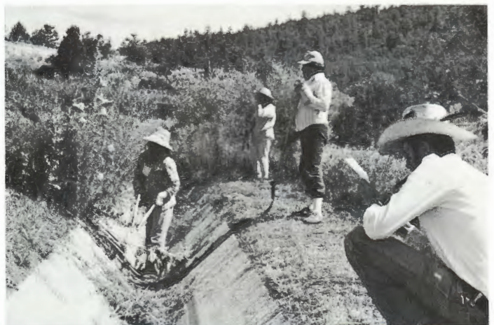
Emergency Jobs Act-funded repair of irrigation ditches on the Confederated Tribe of Warm Spring Reservation, Oregon.
