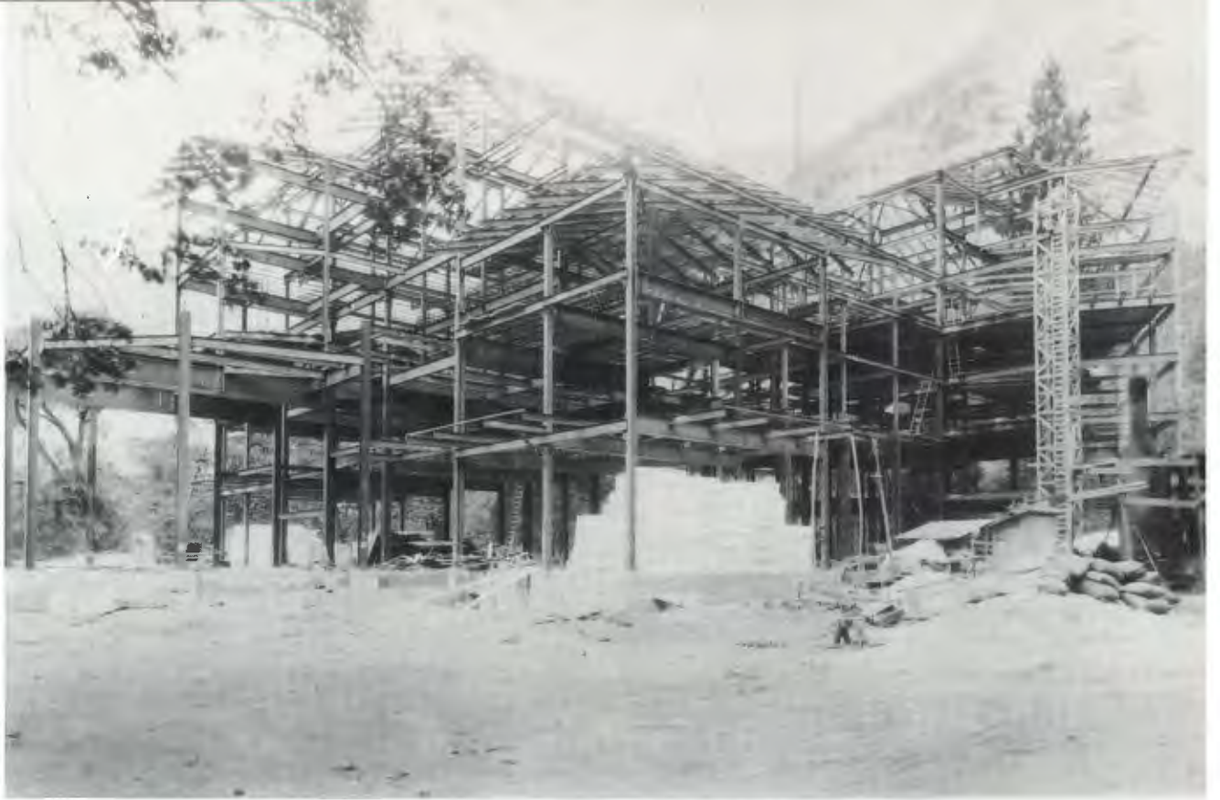
Over 1,000 tons of steel were trucked into Yosemite Valley for use in building the six-story hotel. (Perry Gage Collection.)
